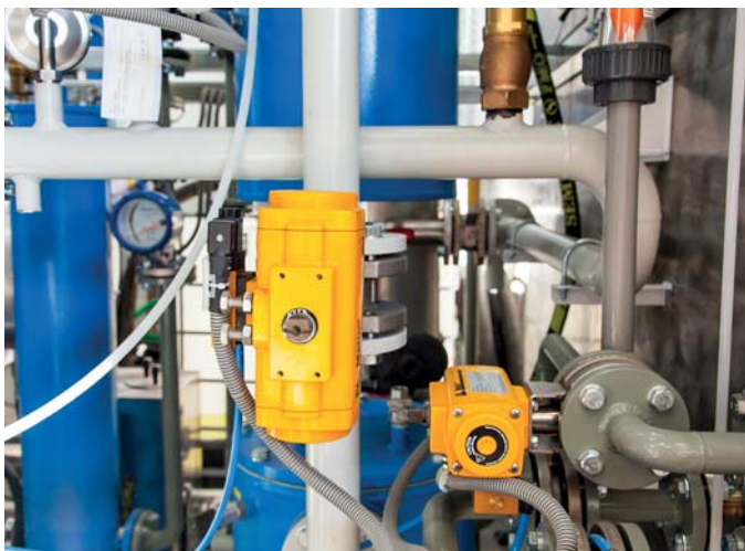
REOIL plant uses highly efficient, fast pneumatic control valves to ensure high reliability of operation throughout the lifetime of the plant.
