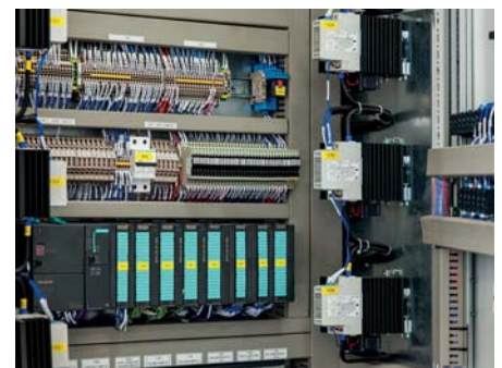
All electrical wiring across the REOIL units conforms to the highest European standards and consists only of high-quality components to ensure the reliability of the unit.
